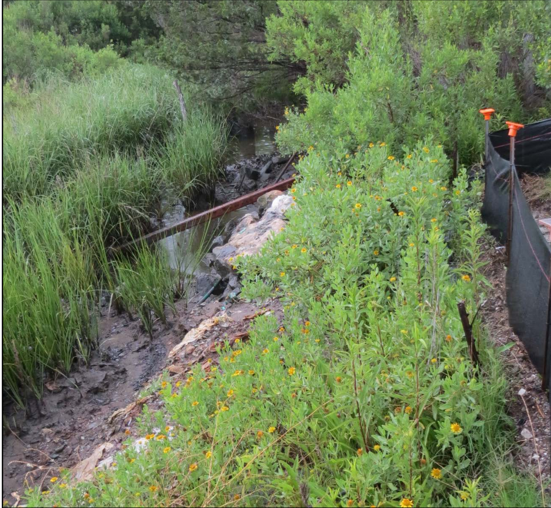
Figure 4. Erosion of municipal landfill cap in Gadsden Creek.
